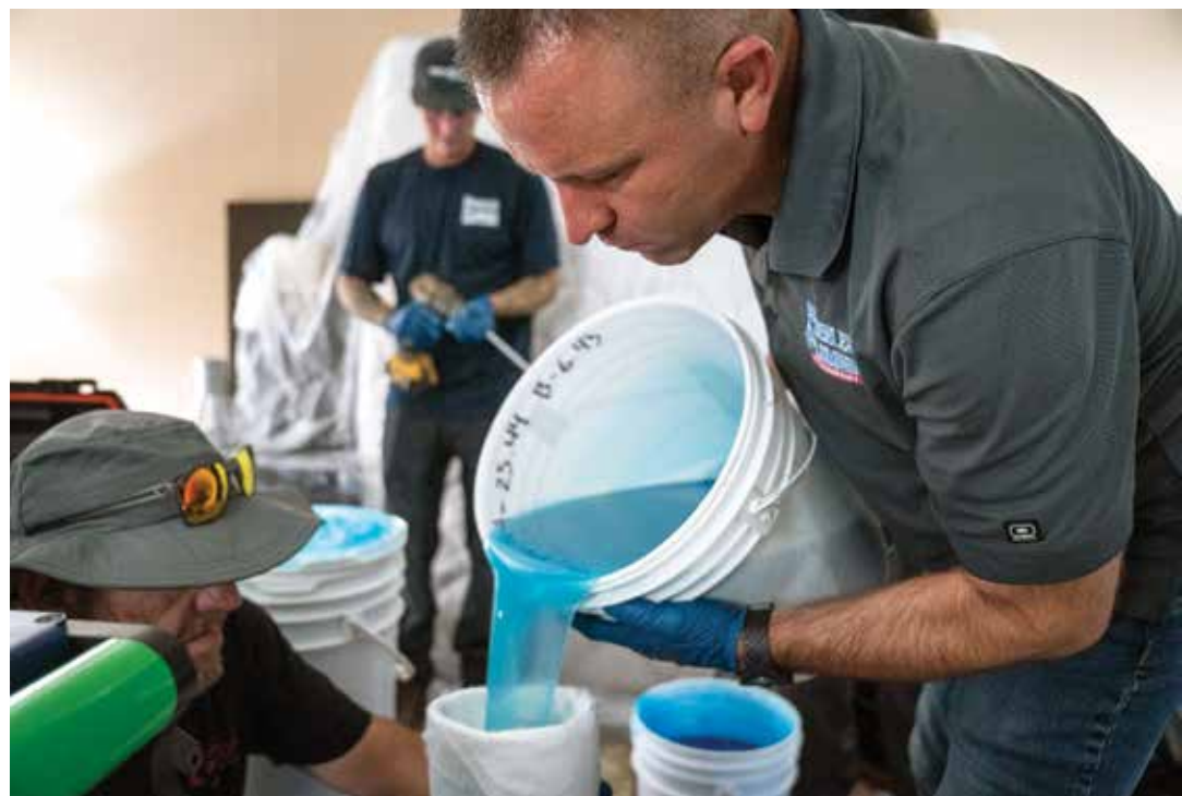
» Christian Rushing pours epoxy during a sewer rehab job at the SureStay Hotel in Phoenix.
