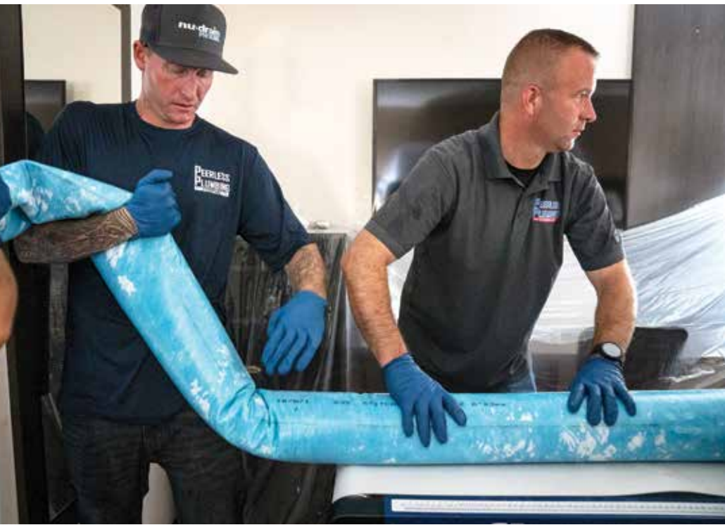
« Michael Eppich-Green and Christian Rushing run liner through the calibration table during a sewer rehab job at the SureStay Hotel in Phoenix.
