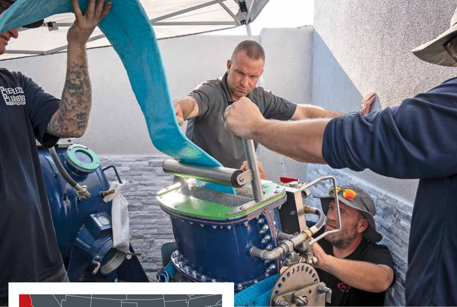
Christian Rushing and crew perform inversion lining on a sewer rehab job at the SureStay Hotel in Phoenix.
